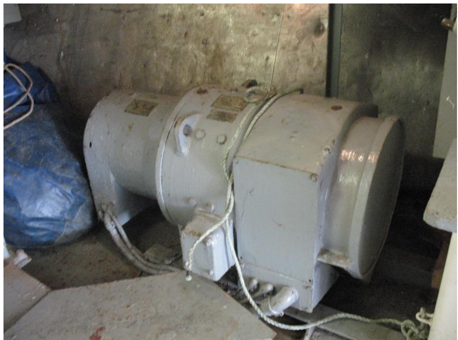
Figure 12: Windlass MG set in foc'sle
