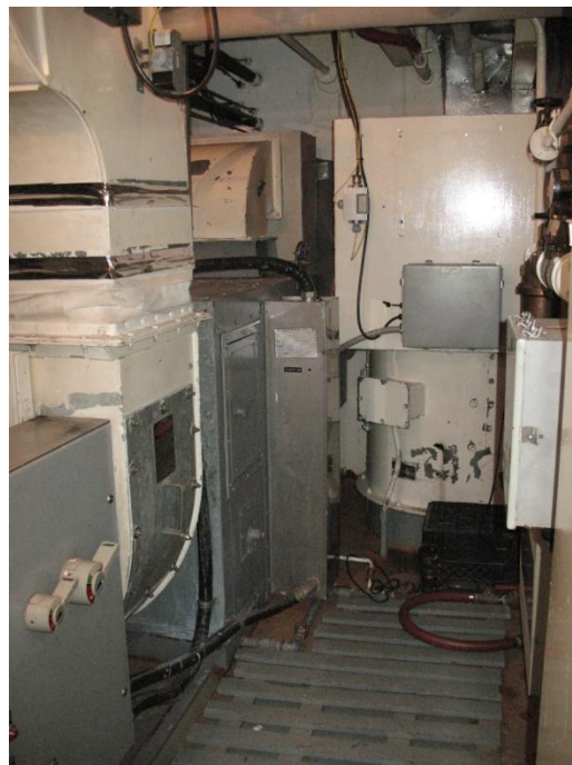
Figure 32: Fan room, typical
