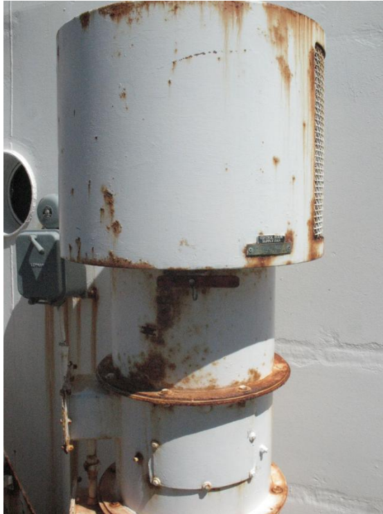
Figure 7: Typical ventilation fan and inlet head
