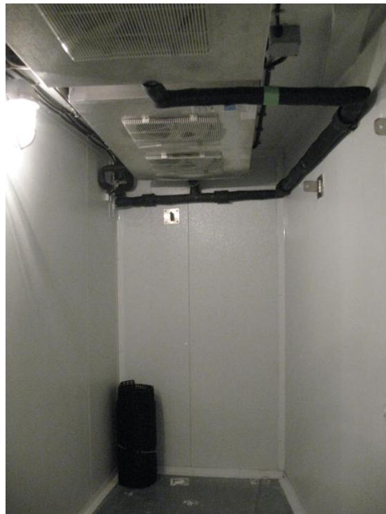
Figure 30: Cold stores locker
