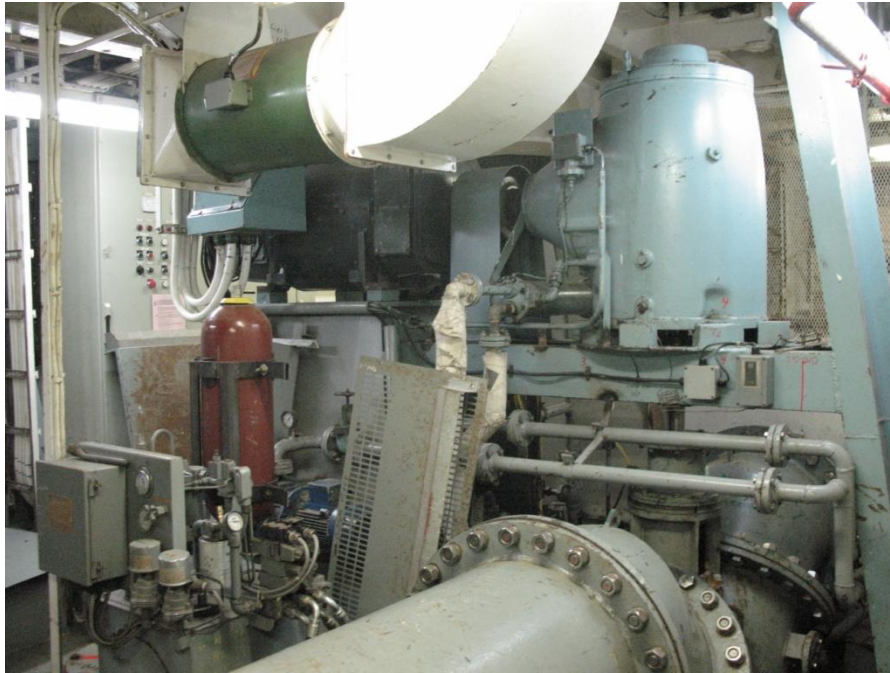
Figure 17: Bow thruster compt.---motor, right-angle drive, control cabinet, discharge tubes
