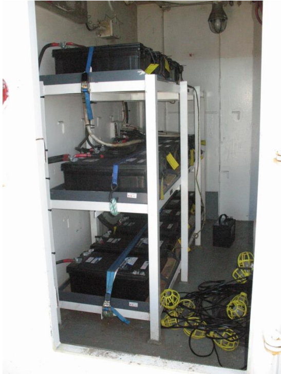
Figure 31: Battery room, boat deck
